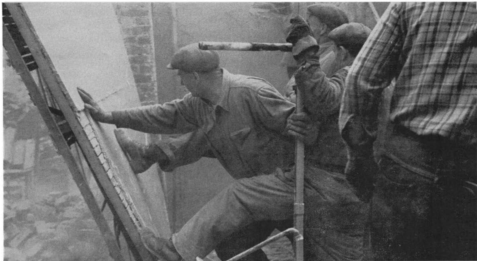
WRECKING CREW moves in to kick and batter down wall after worker at left has softened it up with crowbar.
